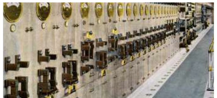
"The largest direct current control board in the world, in the Ford power house." Postcards showing the Ford plant in 1917.
